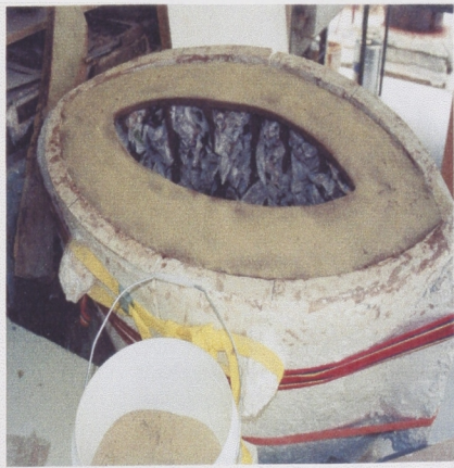
Fig.39 After attaching the base for footing, sand is sprinkled to minimize shrinking cracks during the drying process.
